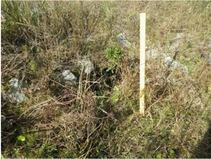
Figure 9. Outlet Location of Damaged Stormwater Culvert
