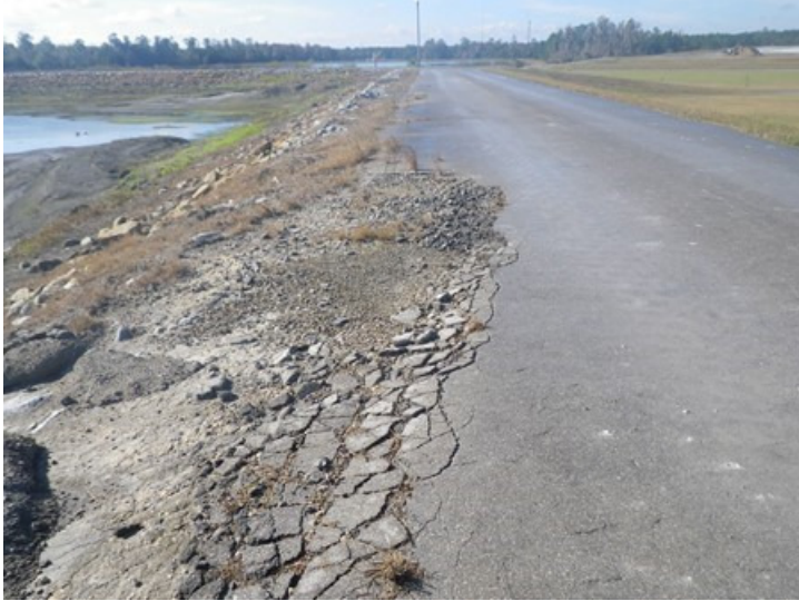
Figure 5. Pavement Damage on the Inside Edge of the Road on the Northern Corner of Ash Cell #1
