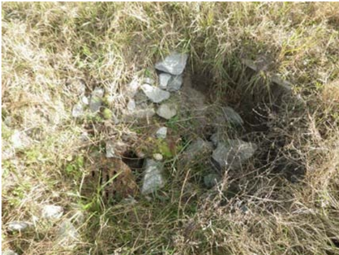
Figure 8. Inlet Location of Damaged Stormwater Culvert
