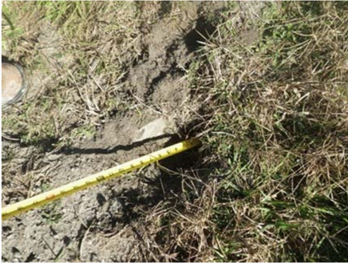
Figure 7. Surficial (<8 Inches Deep) Animal Digging Found on External Western Side Slope
